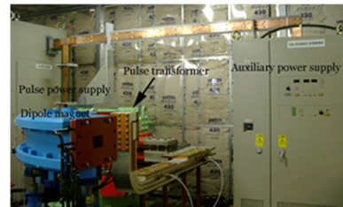
Figure 4: Auxiliary power supply has been connected to the pulse power supply in parallel at the primary winding of the matching transformer.
