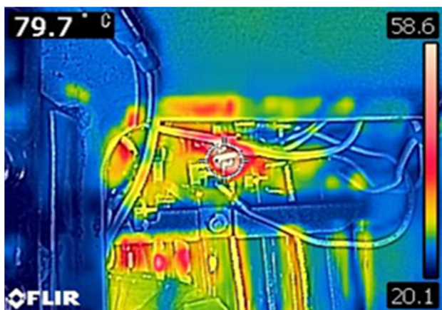
Figure 5: Thermo camera image of magnetic channel.
