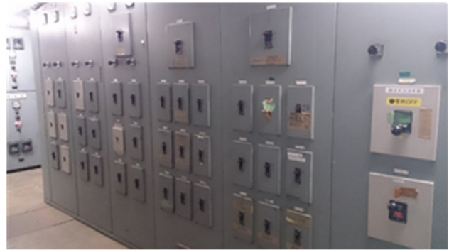
Figure 2: Old NFB and power board.
