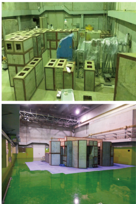
Figure 4: Renovation of wall and floor in the Exp. Hall #1. Upper picture shows an end part of the beam line in the experimental hall before the renovation. Lower picture shows the reconstructed shield blocks after the renovation.
