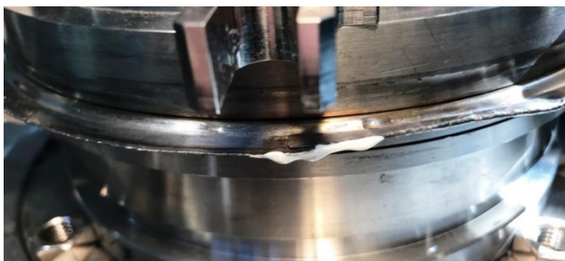
Figure 8: TORR SEAL (Agilent Technologies Part Number 9530004) applied to one of the leak points.
