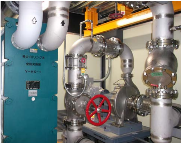
Figure 8: Heat exchanger, Pump & Motor and Overhead Rail.
