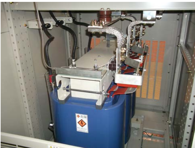
Figure 6: Double power Transformer
