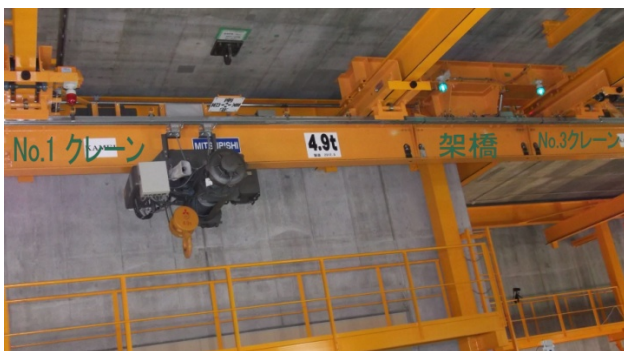
Figure 3: Hoist, crane beams, and transfer-bridge.
