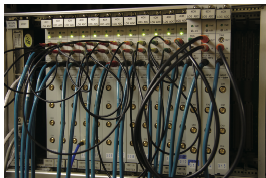
Figure 12.79: 18K11 L/R detectors in a VME64x sub rack.
