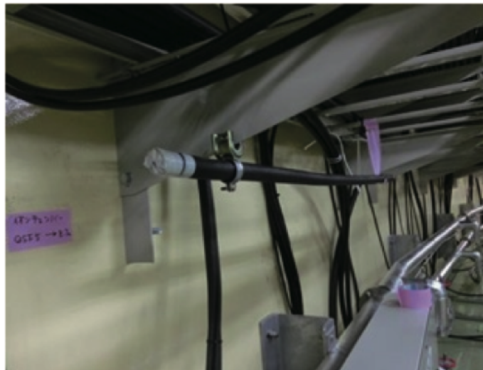
Figure 12.93: Ion chamber that mounted on the cable rack.
