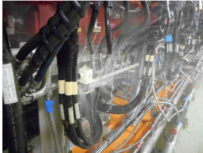
Water leakage from old flow sensors
