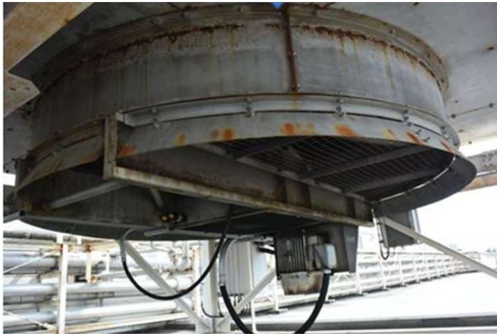
Erosion of Klystron cooling towers
