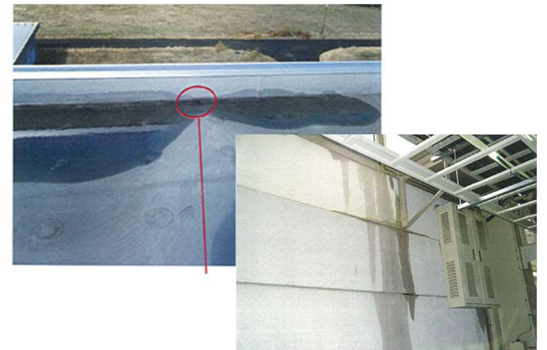
Leakage of roof of power supply buildings
