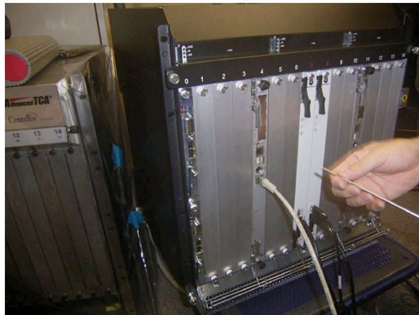
Redundant switch fabrics
